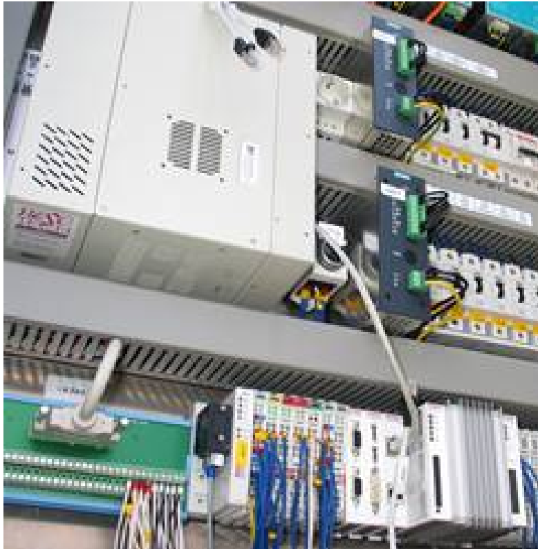
Figure 15: Transformer monitoring and merging unit IEDs
