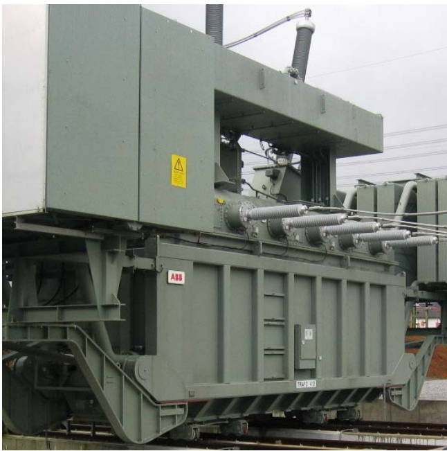
Fig. 7 Transformer T412 in Nehden
