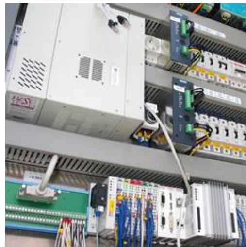
Fig. 12 Transformer monitoring and merging unit IEDs
